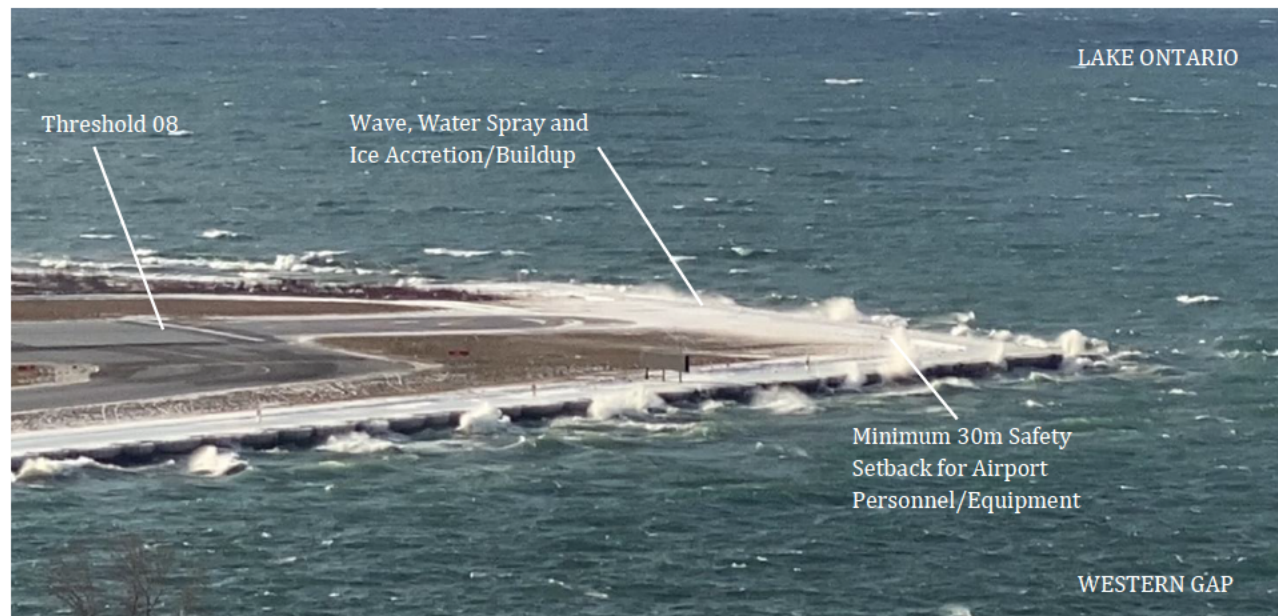
Figure 18: Water Spray and Ice Buildup on Western Seawall (Threshold 08)
